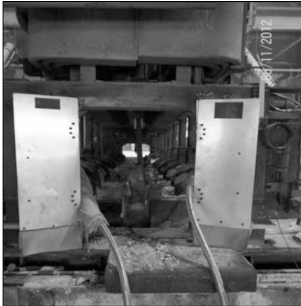
Figure 6. Center channel at end of bake cycle. High-temperature steel hoses connect aluminum pipes to air supply.
