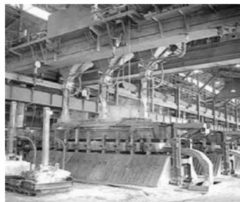
Fig 2. Aluminum smelter pot room being fed of alumina by the multipurpose overhead crane.
