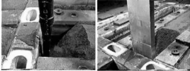
Figure 9 – Albras bake furnace coke suction system before and after modifications – source: [9].
