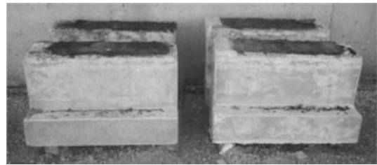
Figure – Old Cross-Over Busbar Supports
