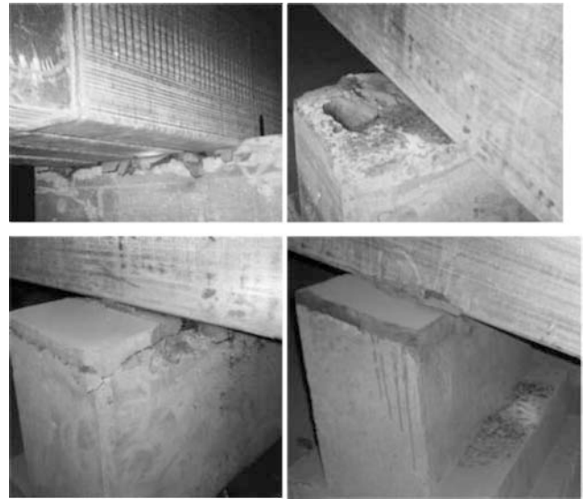
Figure – Typical Cross-over Busbar Supports Before Project
