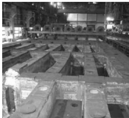
Figure 1 Overview of refractory conditions in furnace 4
