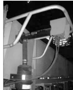
Figure 6 CO analyzer in position on Exhaust Ramp
