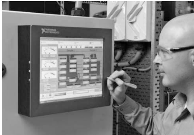
Figure 3. System control via integrated touch screen panel.
