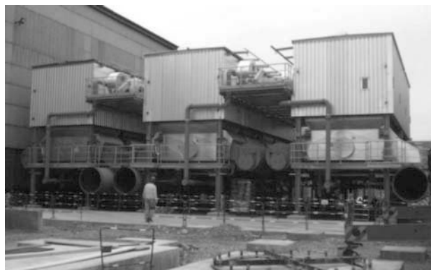
Figure 11: RTO system of a FTS for Several Baking Furnaces
