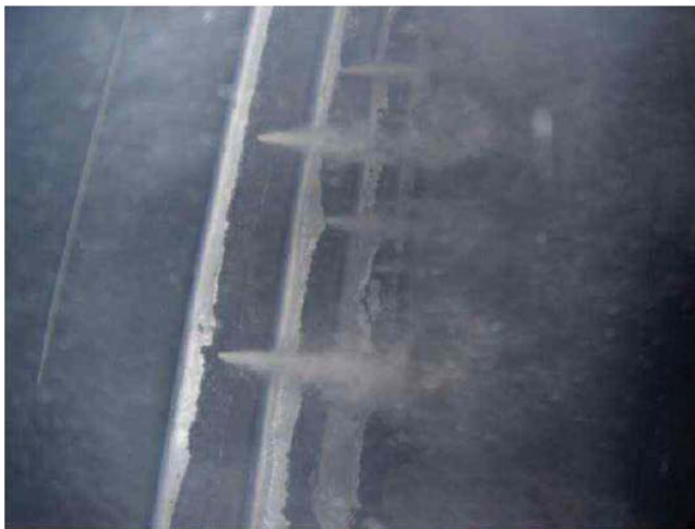
Figure 6: Spraying nozzle operation inside duct
