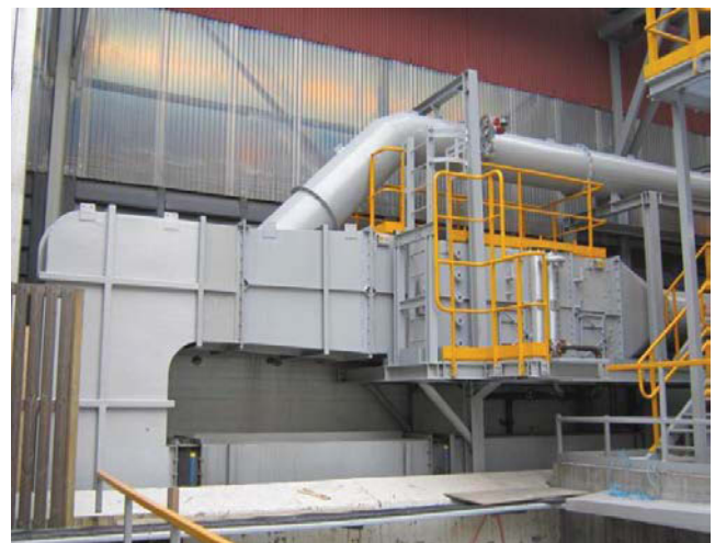
Figure 8: Heat exchanger installed at Hydro’s test center (TOS) in Øvre Årdal, Norway.
