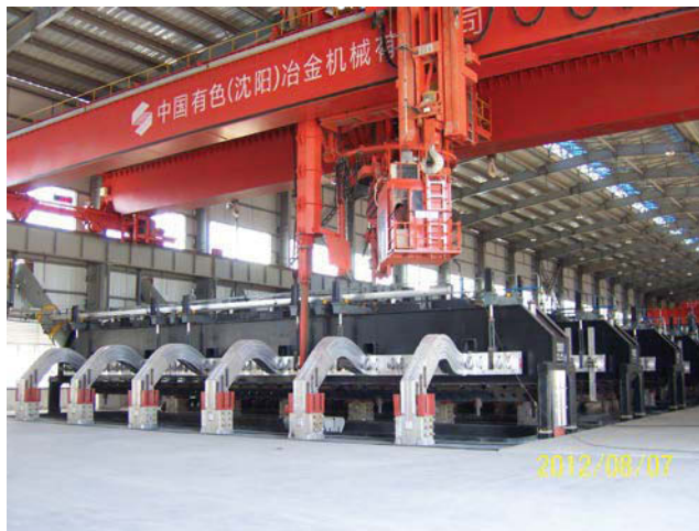
Figure 1a. The 530kA potline (six risers)
