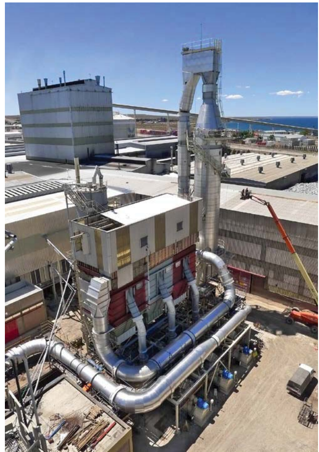
Figure 2: The new FTC in operation
