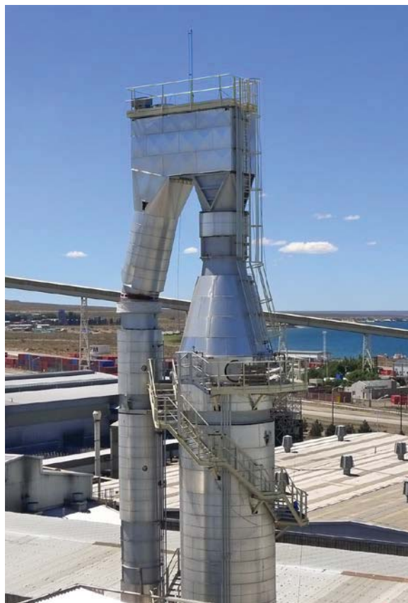
Figure 4: The new Cooling Tower in operation
