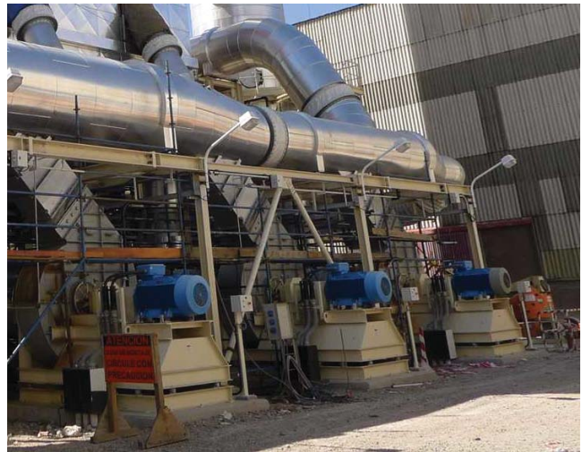
Figure 8: Fan system in operation
