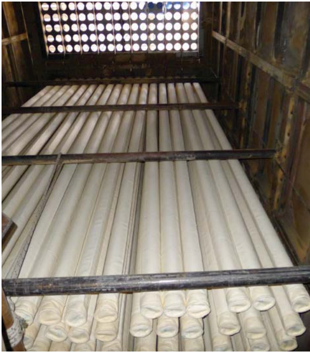
Figure 7: Inner part of the filter chamber
