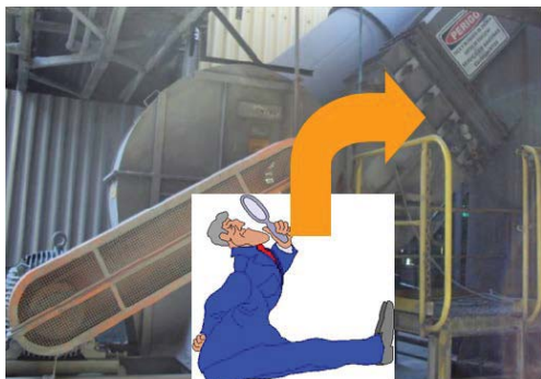
Figure 1 – Exhauster's damper to adjust the volumetric air flowrate of the baghouse.
