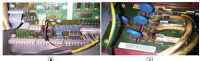
Figure 10 – (a) Disconnected cable in the voltage feedback card, (b) Bad contact in the surge voltage card of the rectifier.
