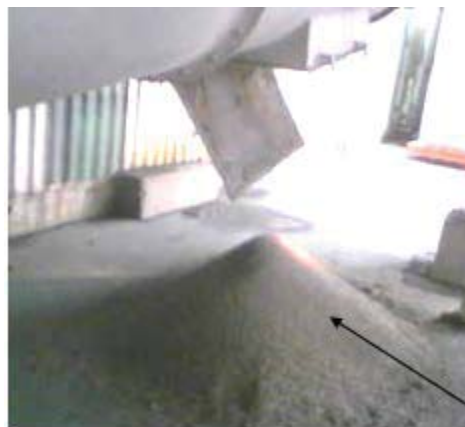
Figure 2 – Clogged pipeline due to lack of intelligent control of the exhauster's baghouse.
