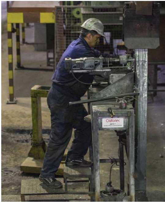
Figure 2: Drill Kit, installed on a platform under the overhead conveyor by-pass loop, for drilling the recess for the RFID tag into the anode rod at AM.
