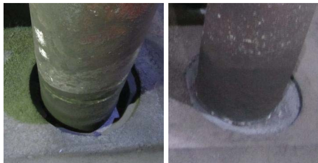
Figure 6. Off-centre position of stub in stub hole and resultant uneven cast iron thimble thickness.
