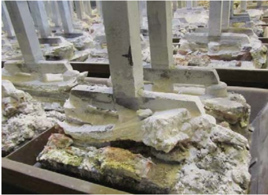
Figure 3. Well maintained end of cycle cover levels, not engulfing the yoke arms.
