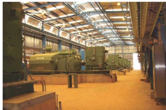
Figure 5. Photo of Pump Station.
