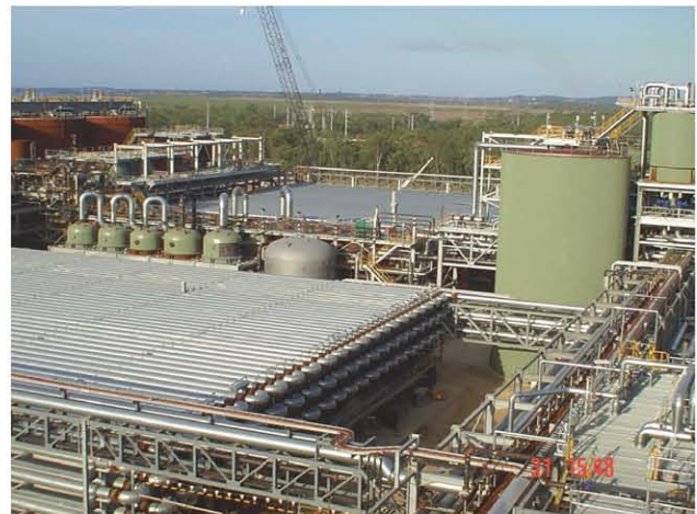
Figure II: The Tubular Digestion Facility at CAR
