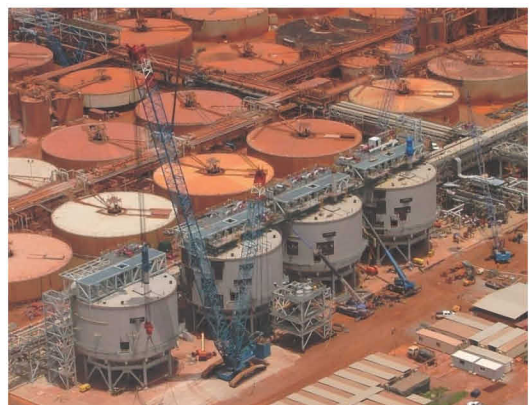
Figure 6. Alcan Deep Cone® Thickeners at RioTinto Gove Refinery.
