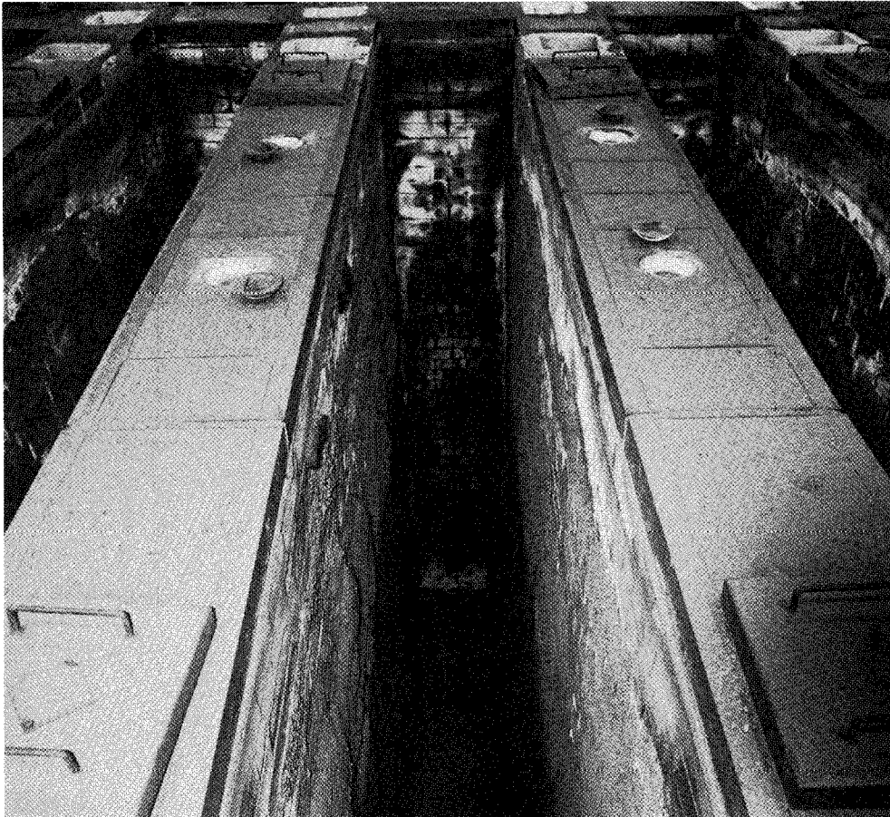
figure 8: Flue according to the "state of the art 1985" after 50 fire cycles
