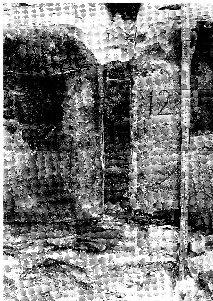
Figure 25. Erosion of the central joint in a cathode with split bottom blocks. Pot life was 595 days.
