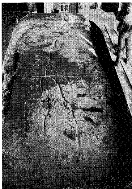
Figure 12. Failed cathode with extensive cracking pattern in carbon lining caused by bottom heave. Pot life was 501 days.
