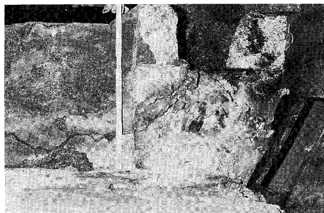
Figure 6. Cathode failure caused by massive bath and metal penetration through shrinkage crack (surface covered with frozen bath and metal) in peripheral seam. Pot life was 5 days.
