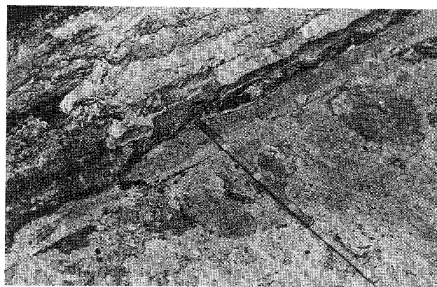
Figure 20. Horizontal extension of carbon bottom (bottom blocks in foreground) due to erosion of ramming paste incline. Pot life was 262 days.
