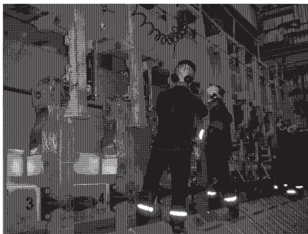
Figure 4: One of 16 anode flex sets being removed with aid of adapted transfer assembly
