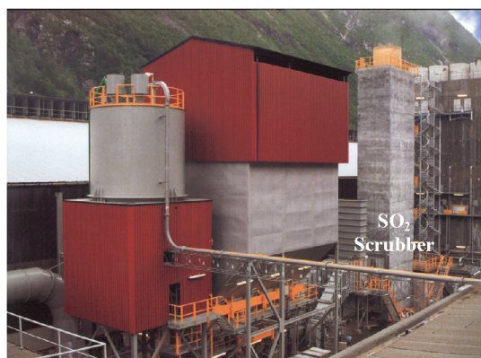
Figure 4. Photo of the dry HF recovery and wet SO 2 removal scrubber at the Årdal smelter.
