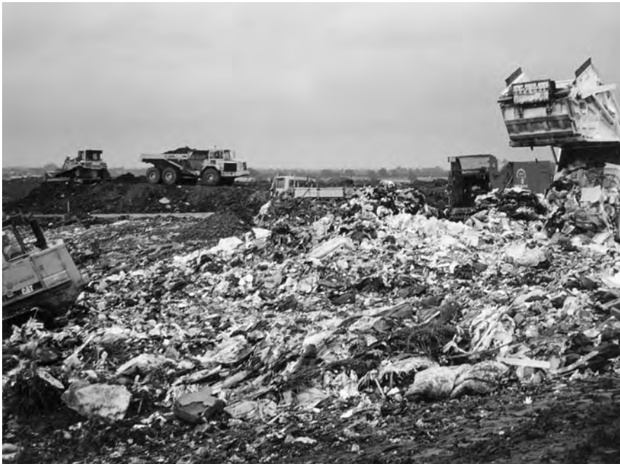
Figure 8.4 The construction of a surface landfill site – Harewood Whin Landfill Site, near York, UK. (Note: The caterpillar tractors spread and compact the waste prior to covering with soil.)
