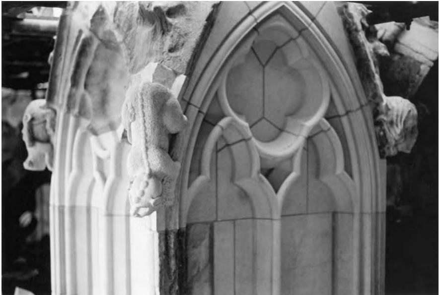
Figure 1.1 Stone erosion York Minster 2000. ( above ) An eroded vestibule buttress on the Chapter House (north side of York Minster). ( below ) The same buttress after restoration.
