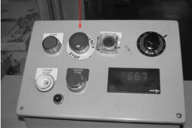
Figure 9.14 An emergency stop button should be located on every control panel. The button should be a red “mushroom” type with a yellow background (arrow).
