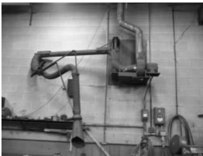
Figure 11.4 Example of local exhaust ventilation equipment.
