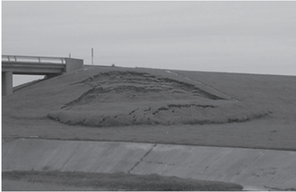
Figure 19.30 Shallow slide in a compacted embankment. (Courtesy of Professor Charles Aubeny, Texas A&M University.)
