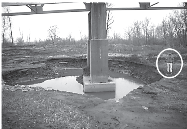
Figure 23.16 Scour hole around bridge pier.
