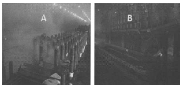
Figure 7: PAHs emissions before (A) and after (B) installing the exhaustion system during anode baking.
