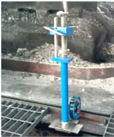
Figure 6: Stand of Interface profile measuring equipment fixed to the pot shell
