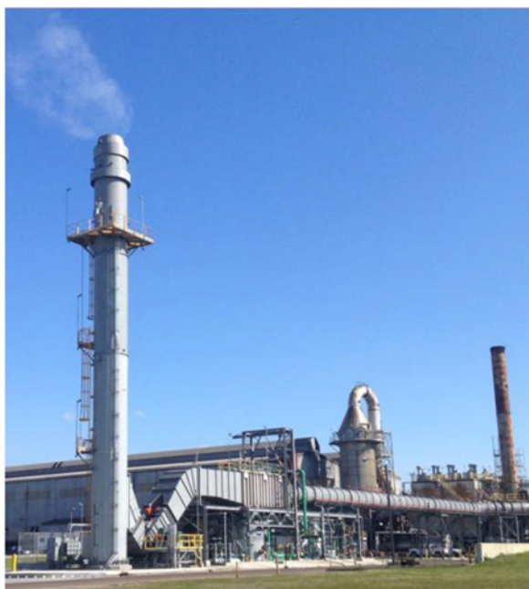
Figure 3. IDS treatment system at Lake Charles, LA facility
