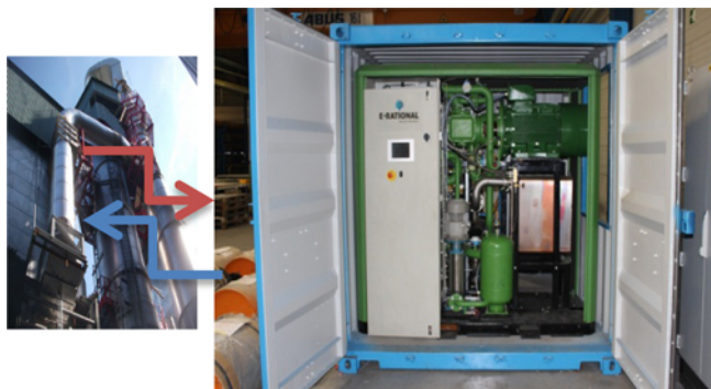
Figure 7: The container size ORC machine connected to the anode bake heat exchanger (AHEx) at Alcoa Mosjøen.
