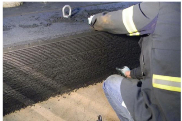
Figure 11. Compaction hardness and homogeneity.
