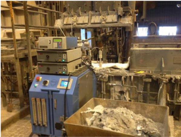
Figure 1. 4 Head Ultra-D degassing system in operation at Southwire alloy rod line
