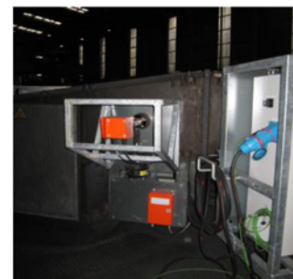
Figure 4. CO Exhaust duct equipped with CO analyzer
