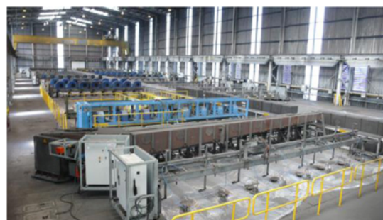
Figure 1. Anode Baking Furnace D at Vlissingen
