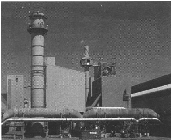
Figure 8 - Dual duct high draft ventilation at Alcoa Deschambault with at the right the smaller, dedicated GTC to handle the extra flows
