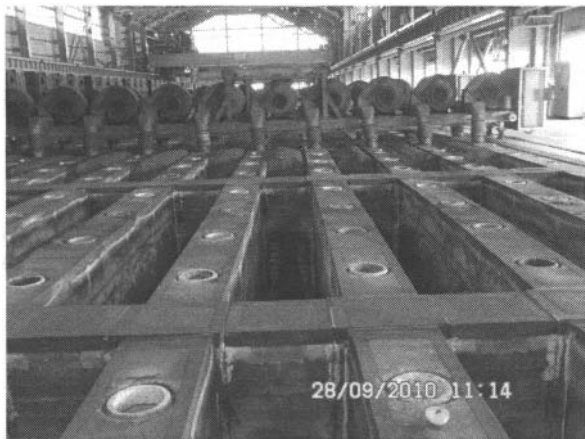
Figure 11 Refractory condition after 40 fire cycles
