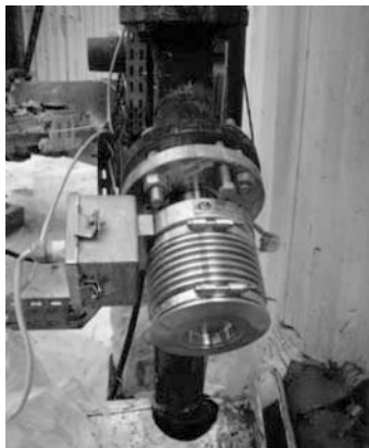
Figure 2 - Refractometer PL&A, model AL-6337, installed online.
