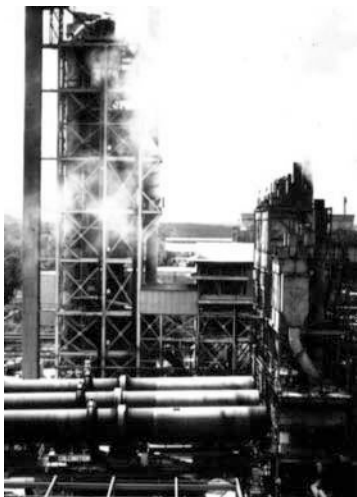
Figure 1. 850 tpd GSC Unit, Hindalco, India.
