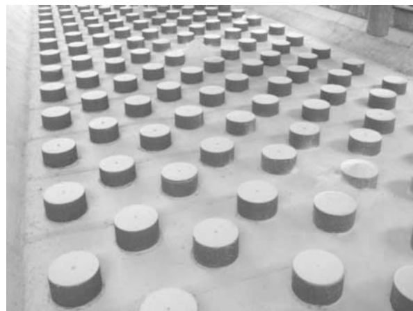
Figure 3: The new generation NSC cells (350kA, in Qingtongxia Smelter)
