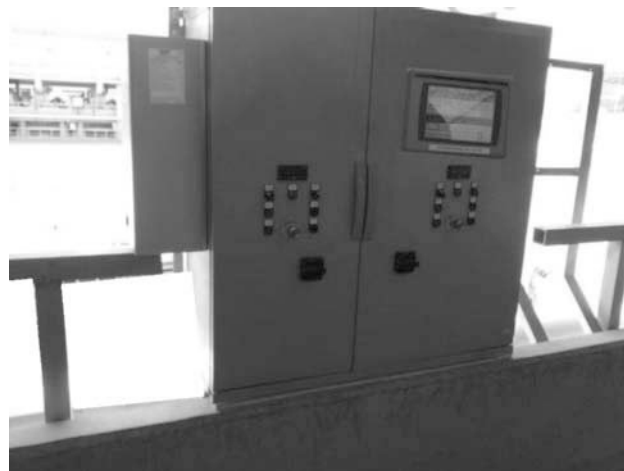
Figure 3. Integrated Pot Control Panel (IPCP) to be installed in EMAL Potline 3.
