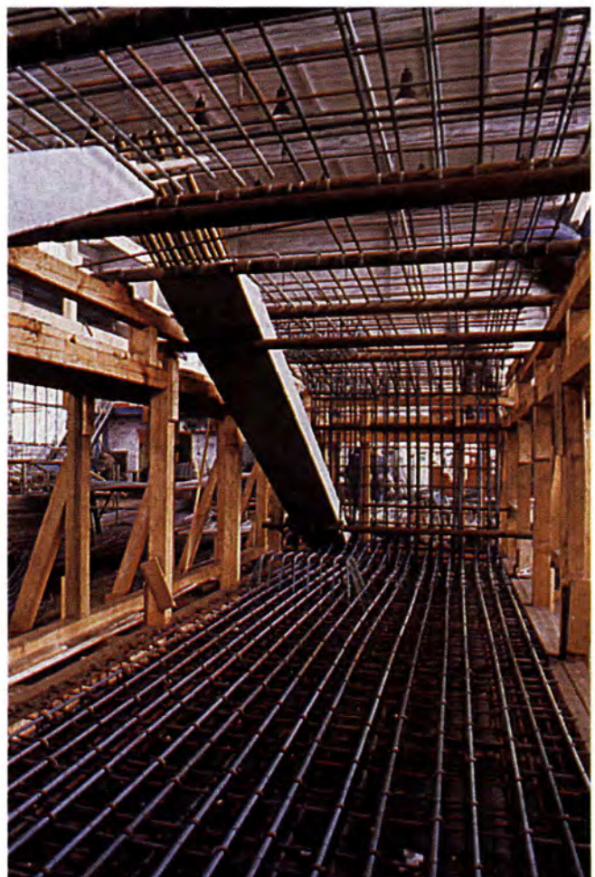
Fig. 25. Elbe River Bridge — reinforcing steel of a typical segment in the wooden template.
