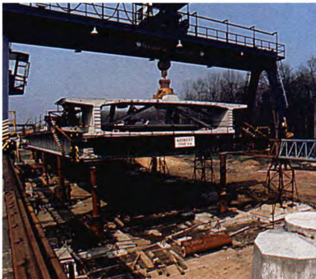
Fig. 27. Elbe River Bridge — erection of a typical segment of the side span.
