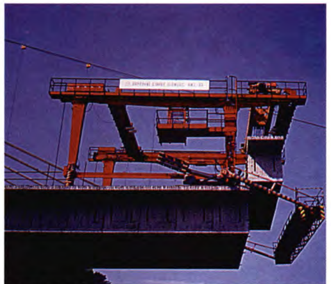
Fig. 29. Elbe River Bridge — lowering of a typical segment of the main span.
