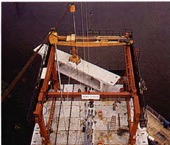
Fig. 28. Elbe River Bridge — turning of a typical segment of the main span.
