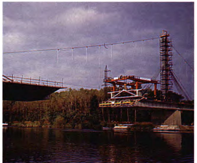
Fig. 30. Elbe River Bridge — erection of a segment of the right cantilever of the main span.
