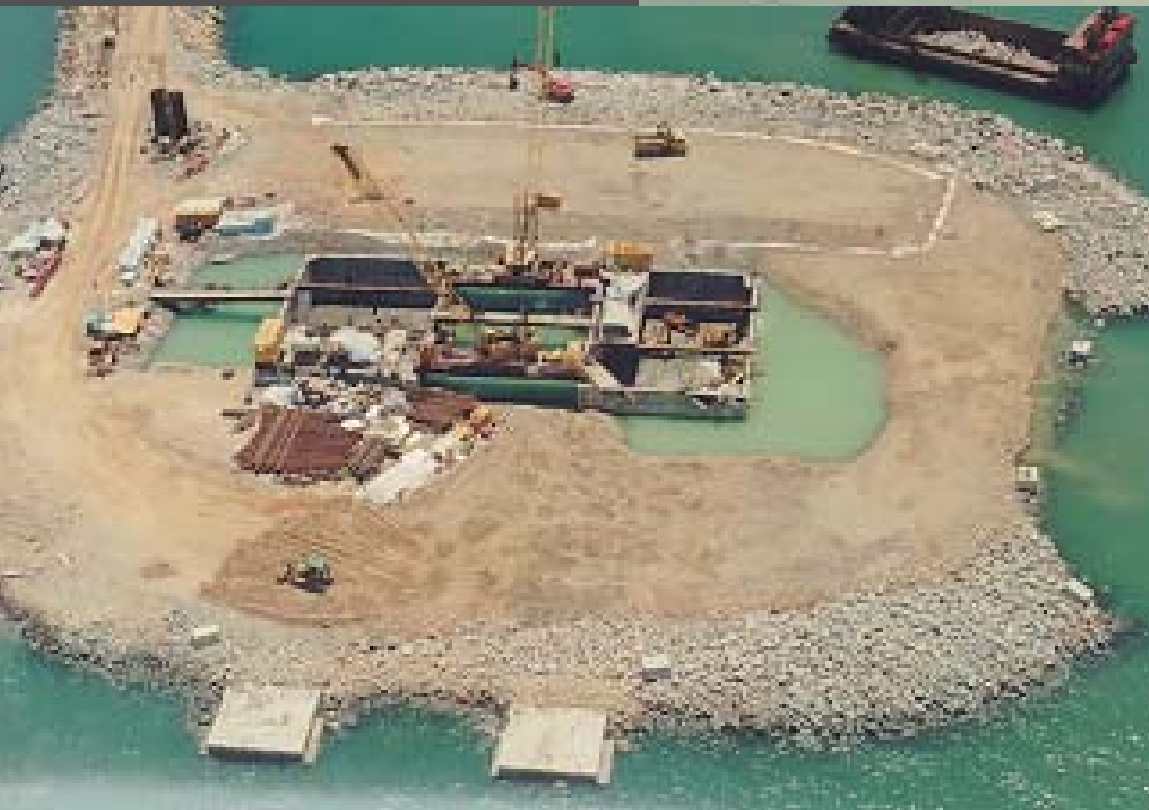
Precast box as footing to bridge tower – Tsing Ma Bridge tower on Ma Wan side
