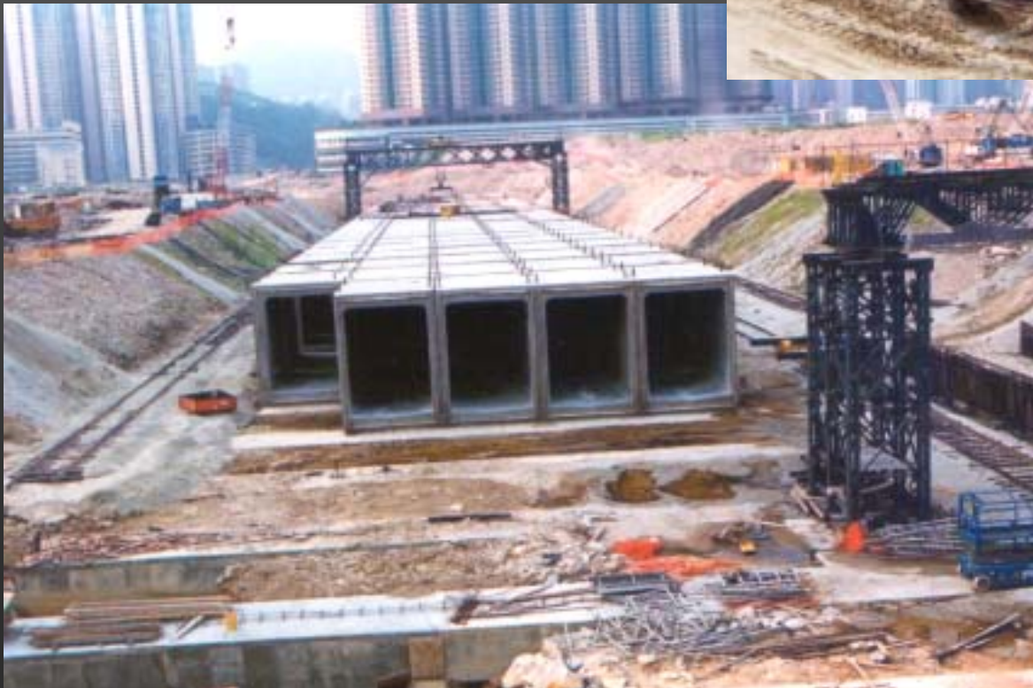
Precast units to form the 4m high 5-cell culvert system in Tseung Kwan O
