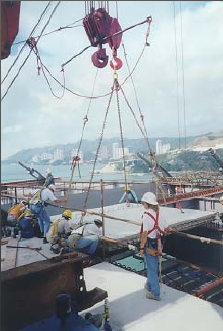
Forming the deck of the Ting Kau Bridge using precast concrete plank
