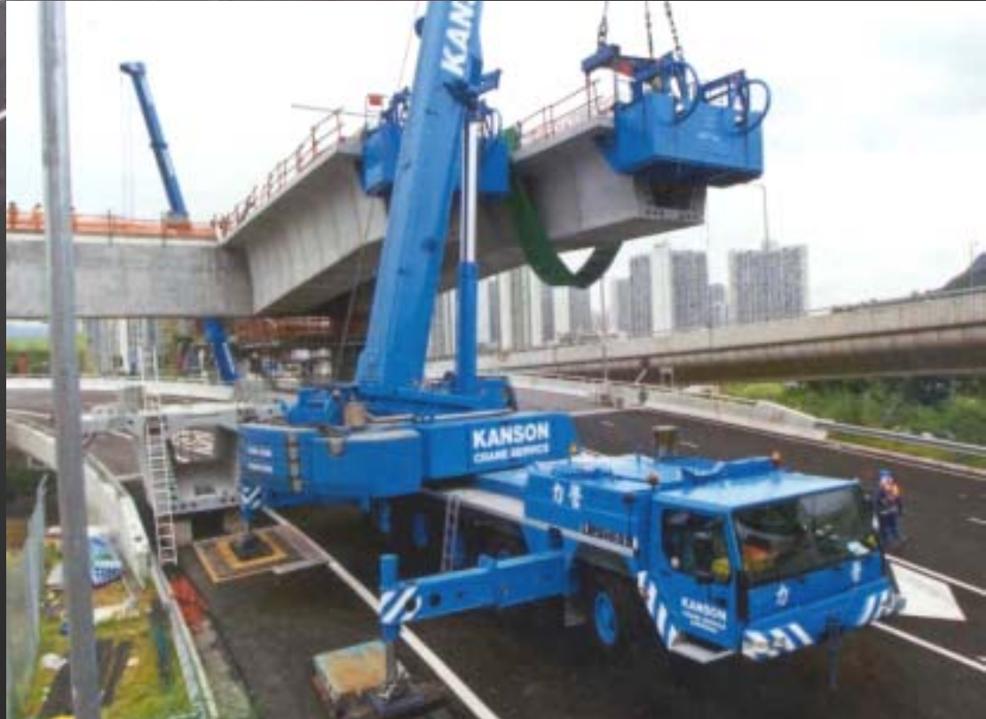
Forming the elevated track of the KCR Ma On Shan Line by precast girder and lifted to deck level for erection using mobile crane
