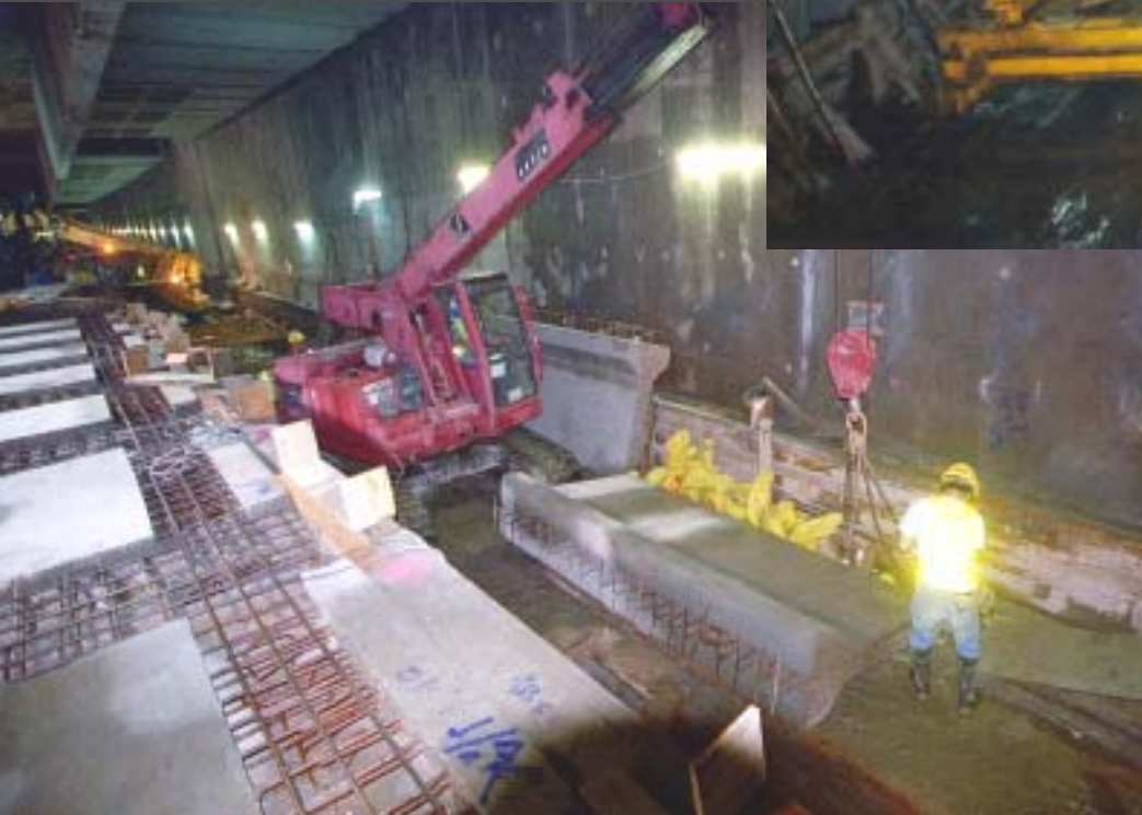
Forming the station platform using precast curb and plank (KCR Tsim Sha Tsui Station)
