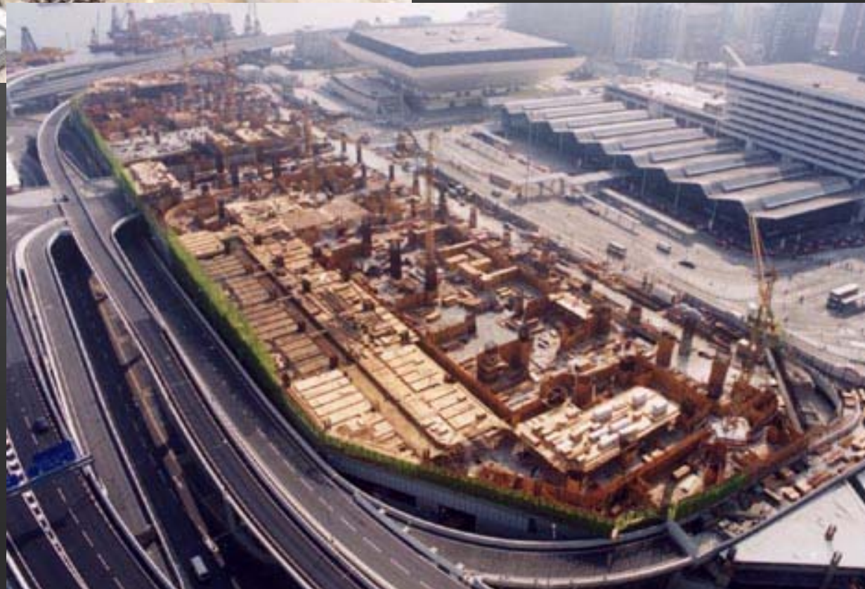
Construction of the Kowloon Canton Rail podium deck – cargo handling bay on the ground level and on top for a large-scale residential development afterward
