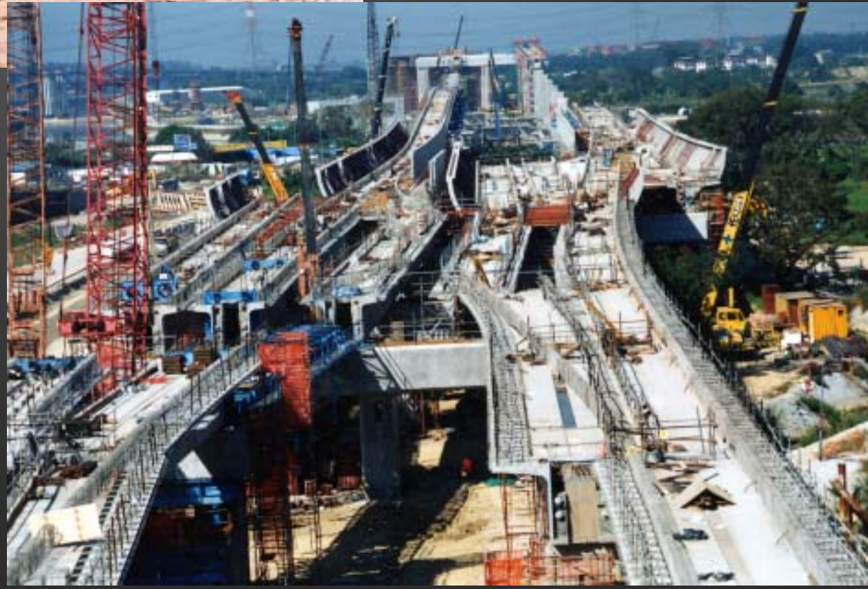
Forming the elevated track of the West Rail using the longitudinal steel support beam
