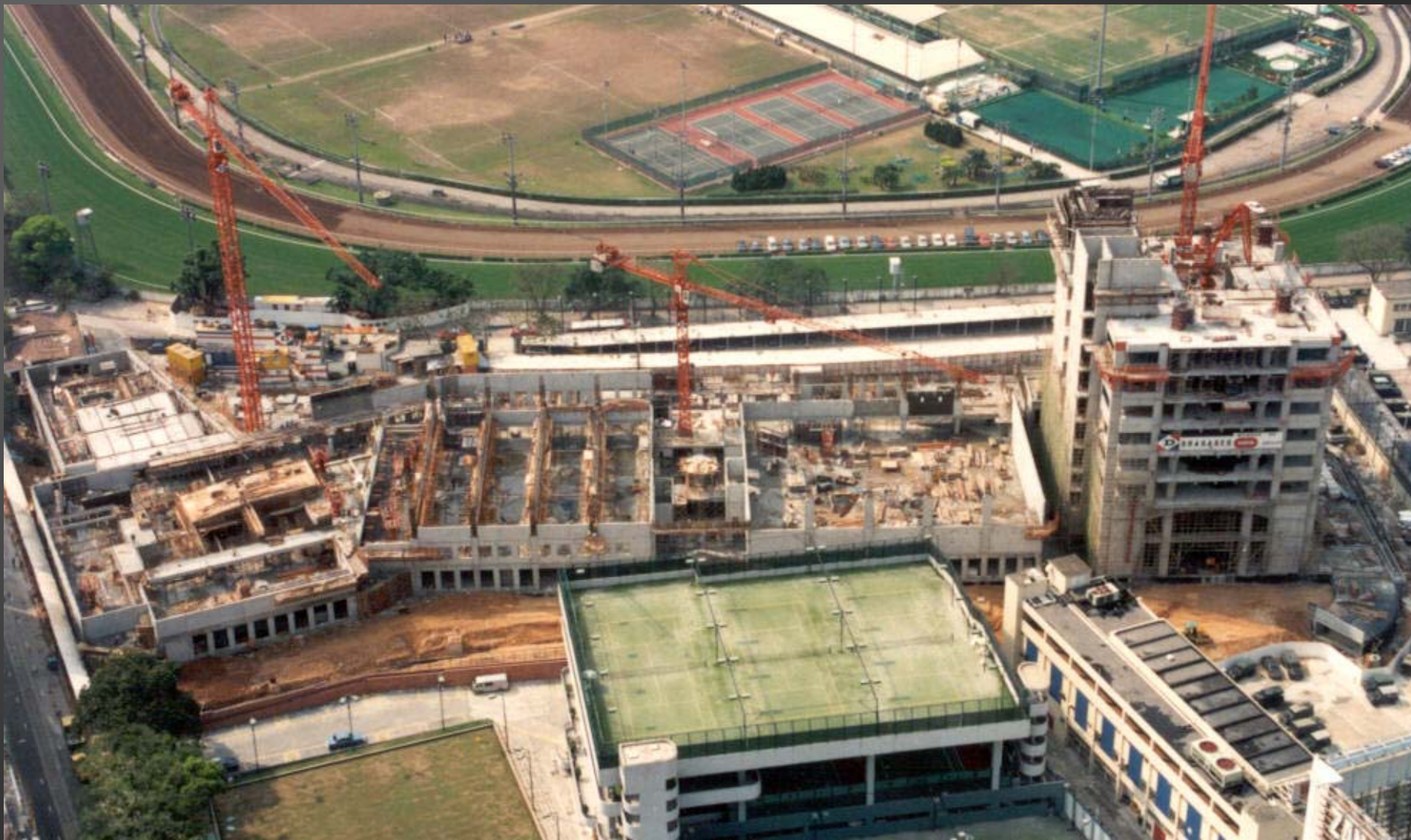
The construction of the Headquarter and Members Facilities Complex for the Hong Kong Jockey Club
